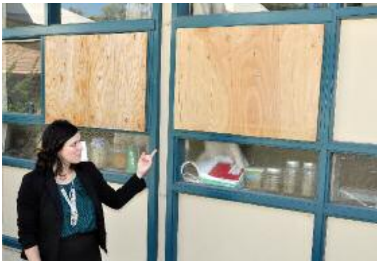
Miramonte High School principal Julie Parks points to boarded windows that were recently broken by vandals at the school.
